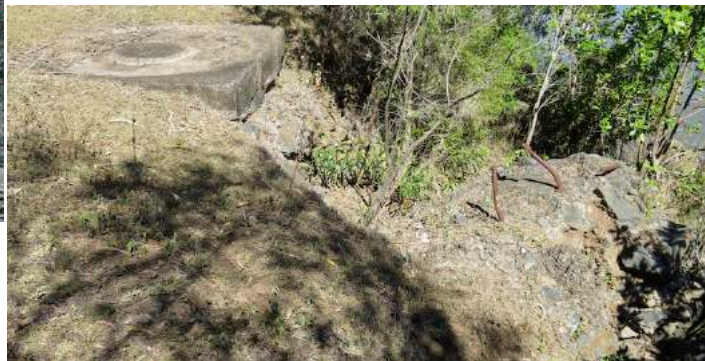
Concrete footings of what could have been the original jetty (Photo © Vaughan Kippers 12:18, 12 th August, 2019)
