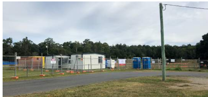
Oxley PDA site showing the start of construction (Photo © Theresa Hoyle 22nd May 2020, 14:29)
